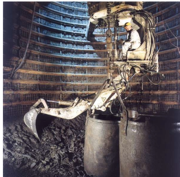
Figure 4: Excavation in unfrozen clay with steel sliding ribs as the primary lining (Oellers and De Bruyn, 1999)
