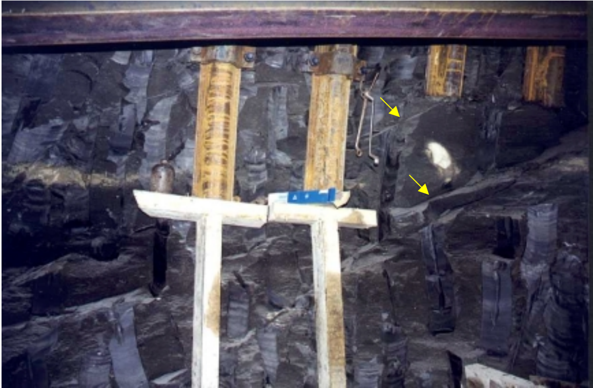
Picture 7: Fractures observed on the lateral wall of the South starting room (1999)
