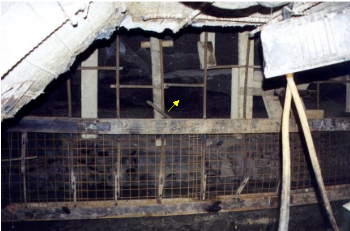
Picture 8: Void created by the detachment of a large clay block at the front of the South starting room (1999)
