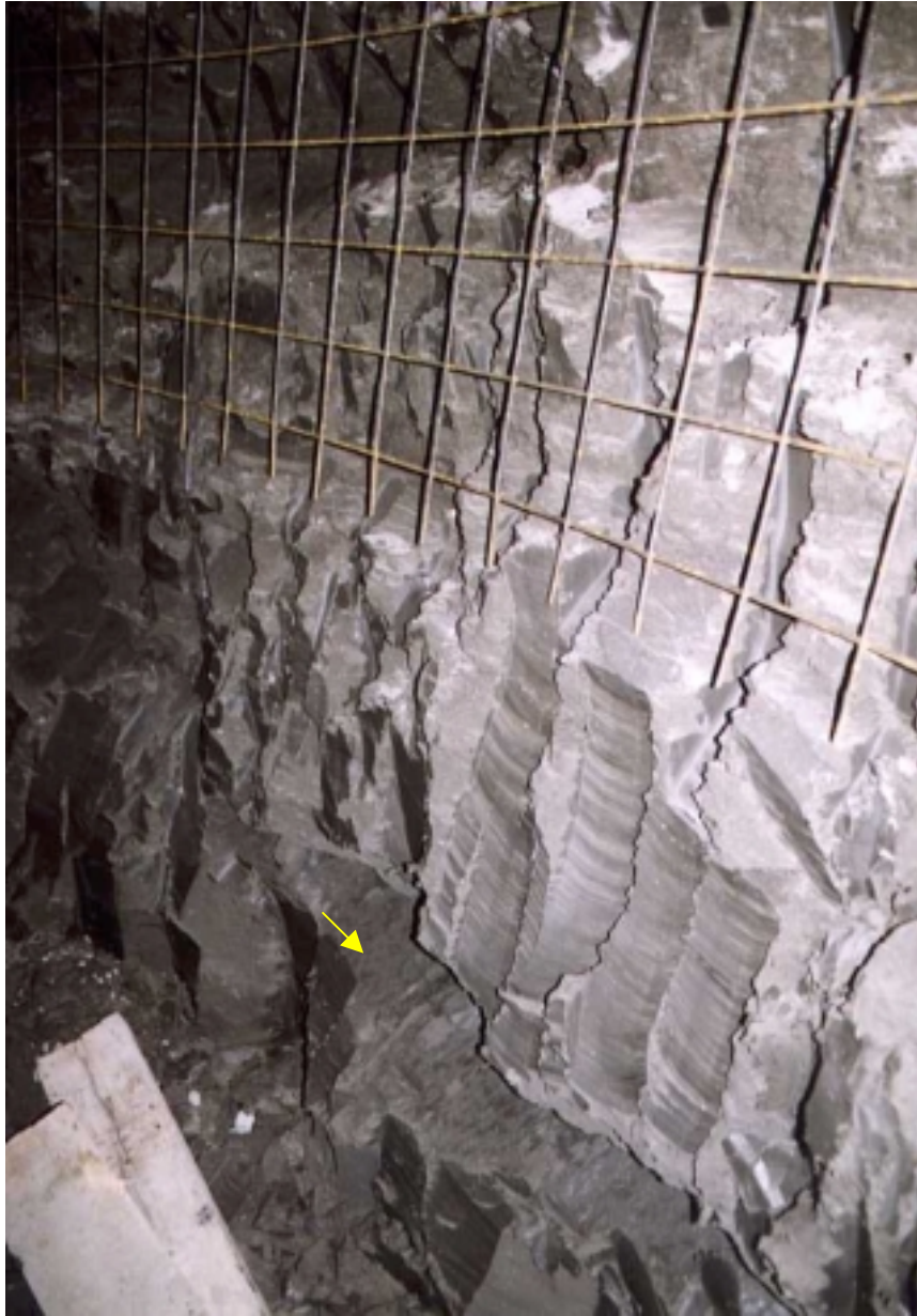
Picture 4: A slickensided surface observed during the enlargement of the foundation (1998)
