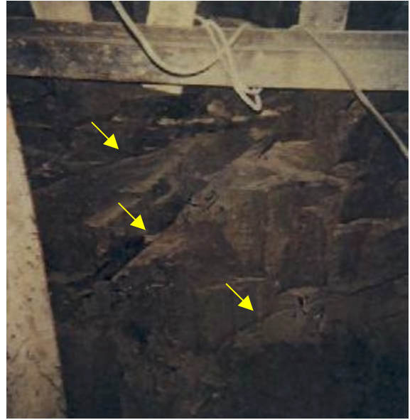
Picture 2: Fracture observed during the excavation of the Test Drift (1987) – West lateral wall
