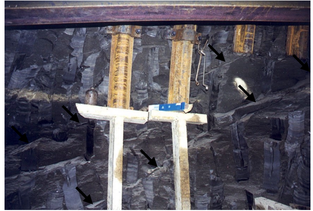
Fig. 5. Traces of the fractures (indicated by the black arrows) in the lateral wall of the South starting chamber.
