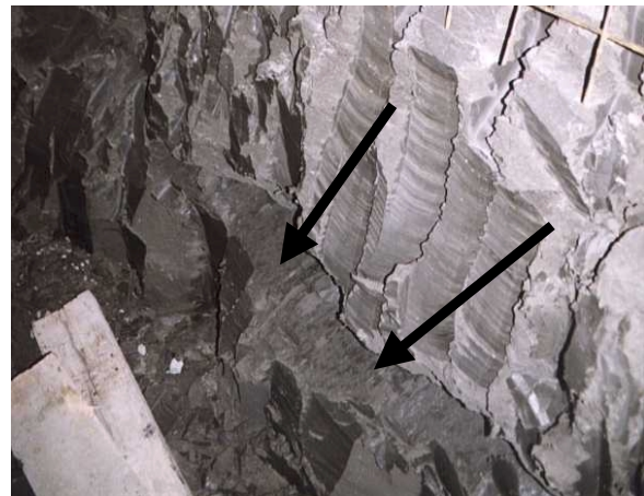
Fig.3. Photograph of a fracture surface in the foundation enlargement of the second shaft.
